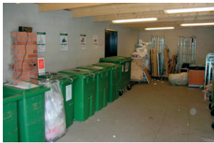
AirMaid® in Waste Rooms
