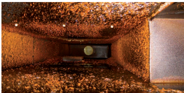
Typical grease buildup without AirMaid results in a high risk for dangerous duct fires and expensive cleaning bills.
