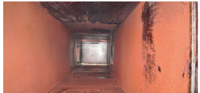
What's possible with AirMaid? A significant reduction or even elimination of grease buildup inside kitchen ducts.
